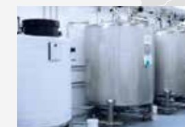
On-site WFI production
